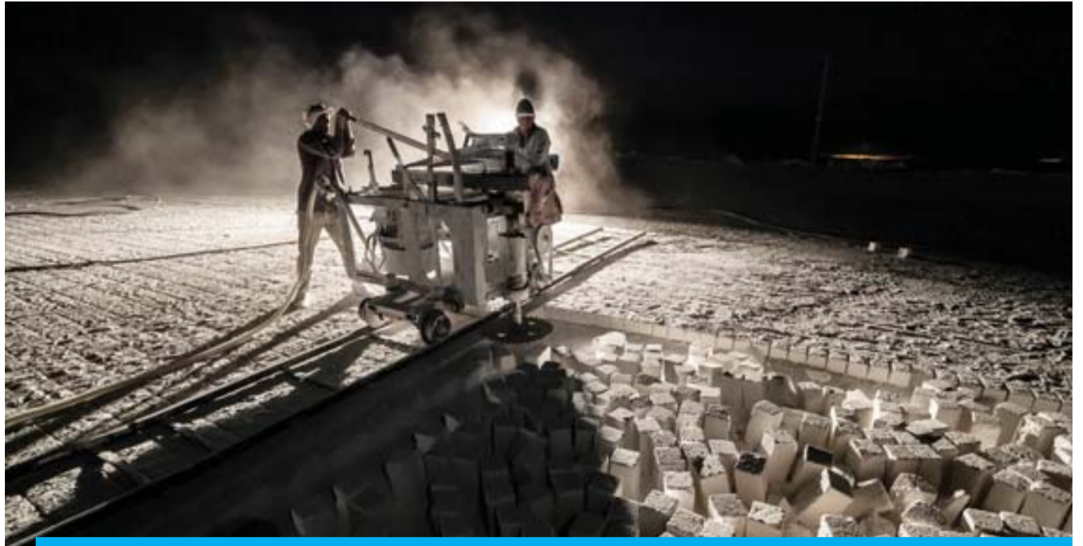
MINYA, Egypt: Laborers work late at the "White Mountain" limestone extraction quarry site near this southern city on Nov 13, 2019. — AFP
