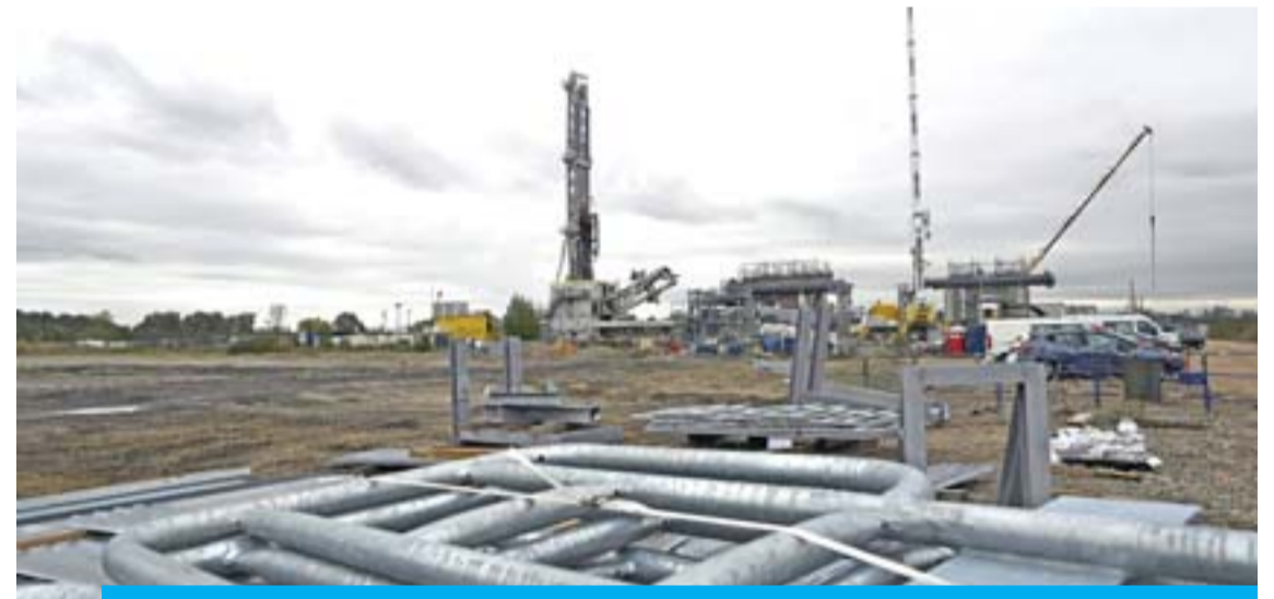
REICHESTETT: Photo shows the deep geothermal well on the site of the former oil refinery in Reichstett, eastern France. — AFP
