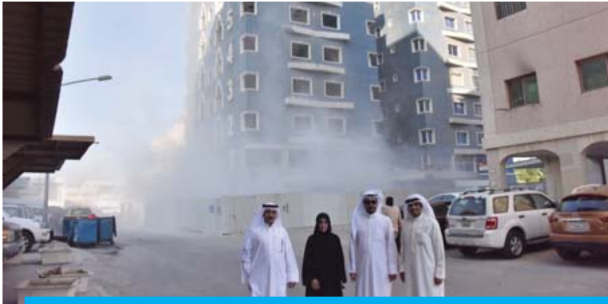
KUWAIT: Kuwait Municipality officials stand as a building in Khaitan is being demolished for violations of construction regulations.
