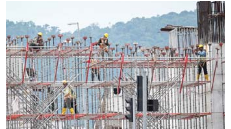
KUALA LUMPUR: Workers set up iron scaffoldings at a building construction site in Kuala Lumpur. — AFP
