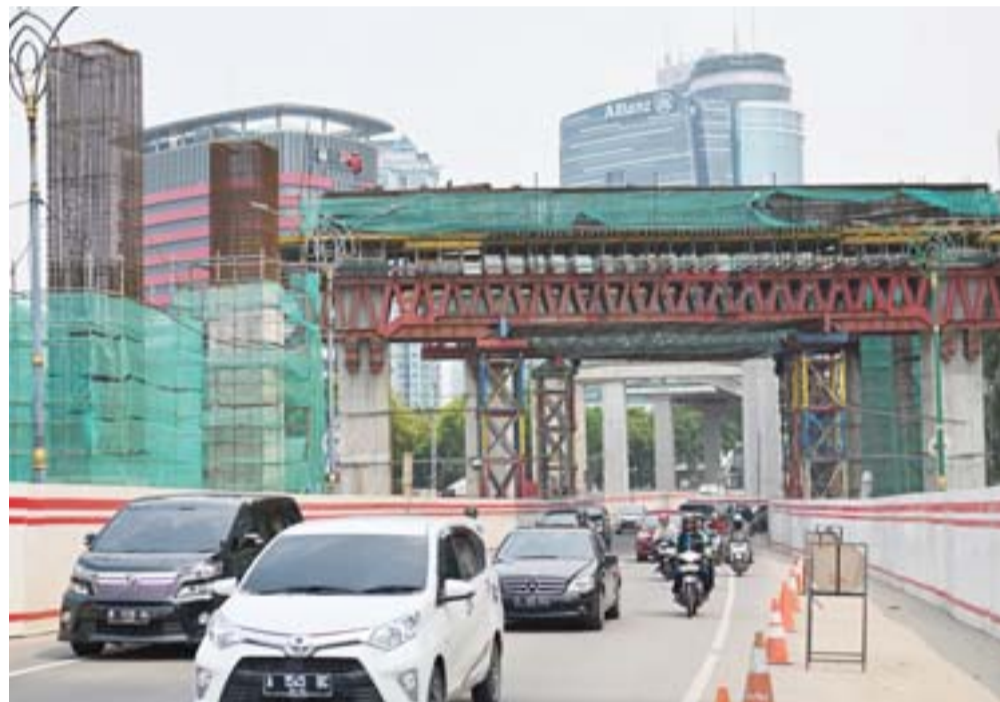
JAKARTA: Traffic travel past a light rapid transit (LRT) construction site in Jakarta yesterday. Indonesia posted another quarter of slowing growth, the weakest pace in two years, as Southeast Asia's biggest economy feels the sting of slumping commodity prices. — AFP
