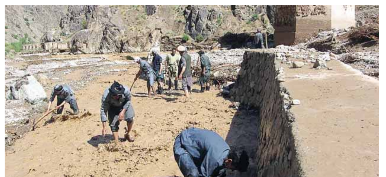
Afghan men working at a site near the Minaret of Jam following floodwaters in the Shahrak District of Ghor Province.
