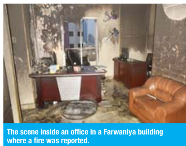
The scene inside an office in a Farwaniya building where a fire was reported.
