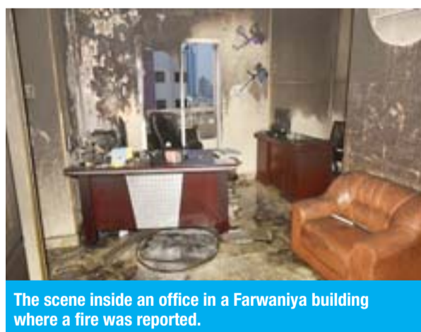
The scene inside an office in a Farwaniya building where a fire was reported.
