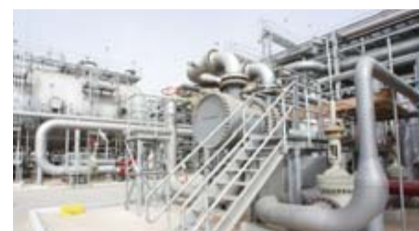
HARADH: File photo shows a general view of an oil plant in Haradh. Two pumping stations on a major Saudi oil pipeline were attacked by drones yesterday. — AFP
