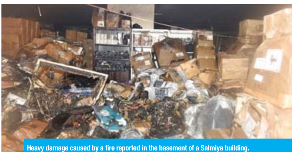
Heavy damage caused by a fire reported in the basement of a Salmiya building.
