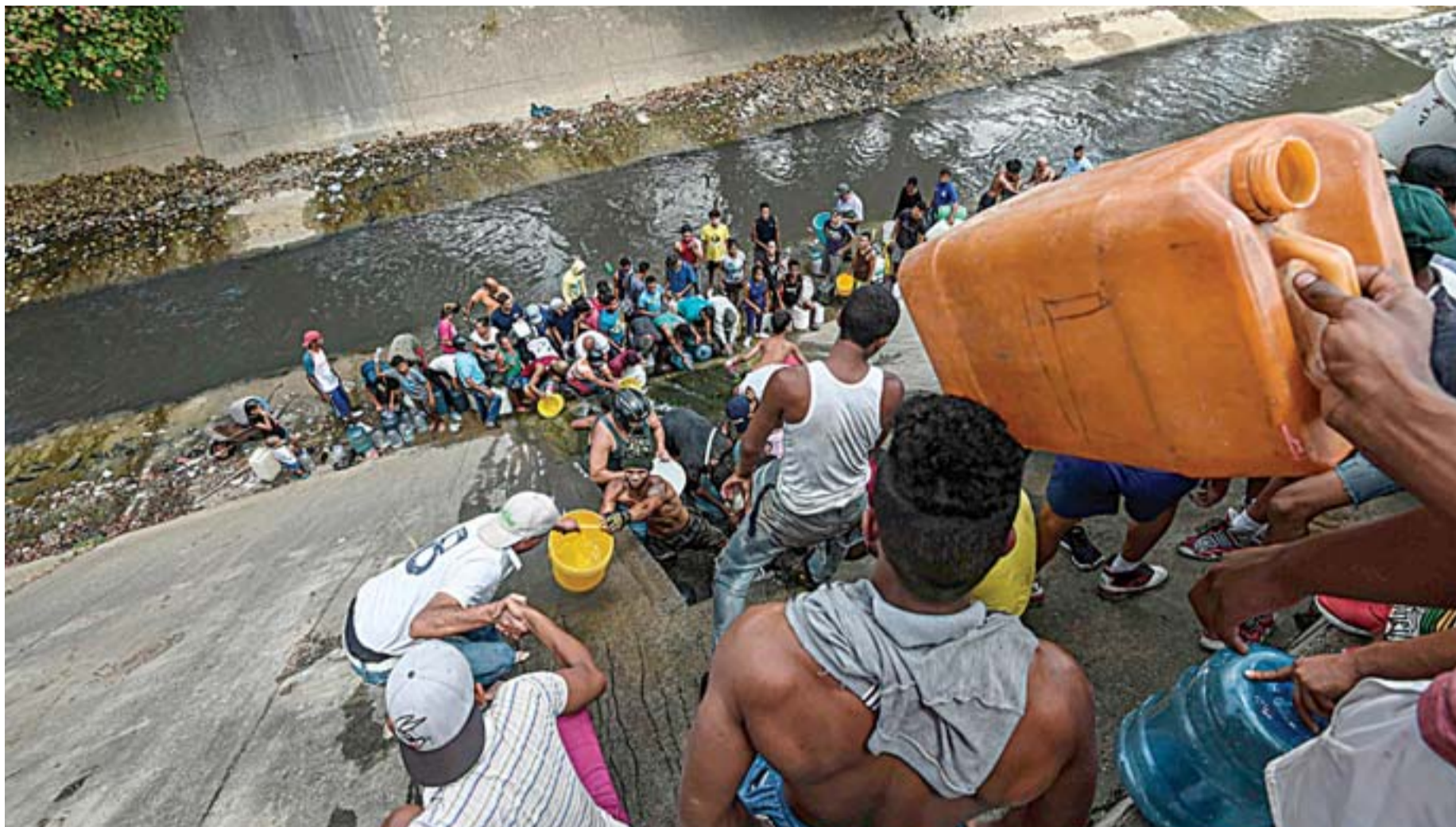
People collect water from a broken pipe, flowing into a sewage canal at the Guaire River in Caracas on March 11, 2019, as a massive power outage continues affecting some areas of the country. —AFP
