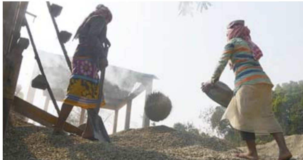
SILIGURI: Indian laborers work in a construction site at the New Chumta Tea estate on the outskirts of Siliguri yesterday. — AFP
