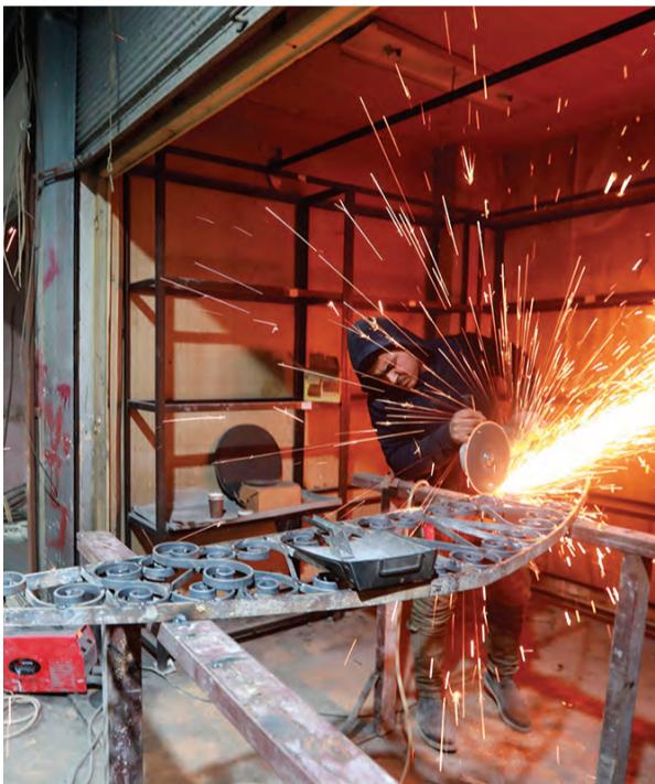
Laborers take part in restoration work at the Saqatiya market in the old quarter of Syria's second city of Aleppo.
