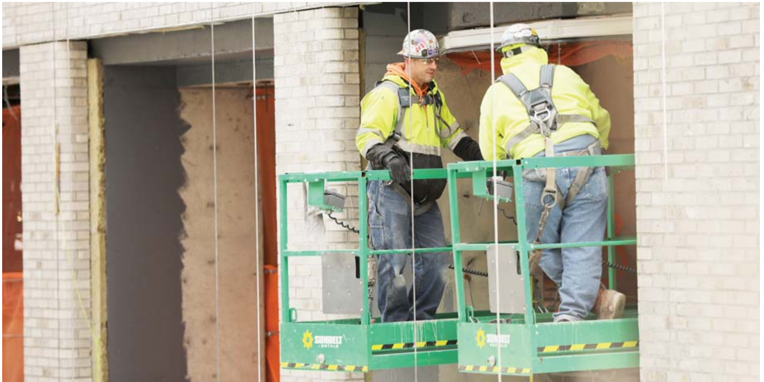
NEW YORK: Construction workers are seen at a building site on Friday in New York City. — AFP
