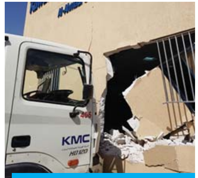
A wall damaged by a truck at a driver's license testing center.
