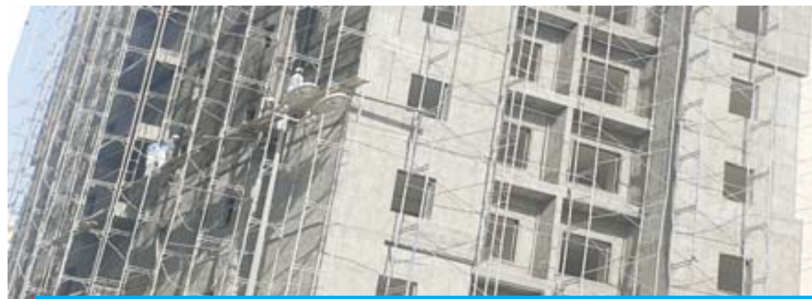
KUWAIT: Workers are seen at a Farwaniya construction site (Block 1, Near Omariya) at 3:00 pm.
