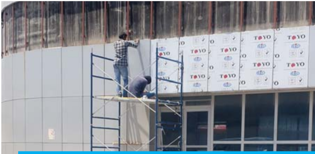
KUWAIT: Workers seen at a construction site in Salmiya. Construction workers continue to work outside, in the direct sun, all over Kuwait despite a ban on working outside from 11am-5pm. — Photo by Ben Garcia (See Page 3)
