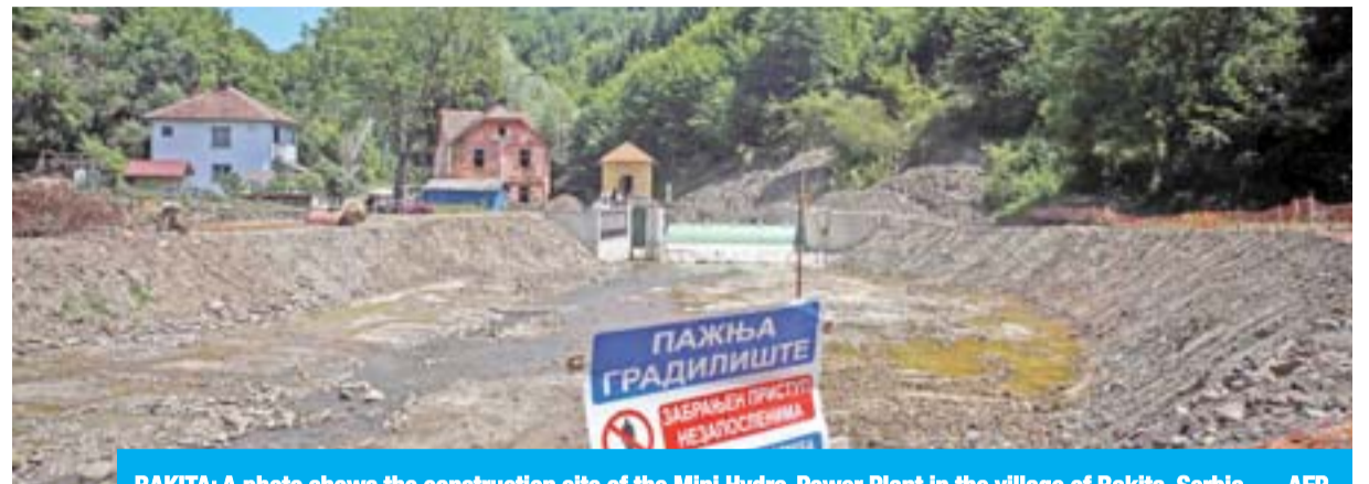
RAKITA: A photo shows the construction site of the Mini Hydro-Power Plant in the village of Rakita, Serbia. — AFP
