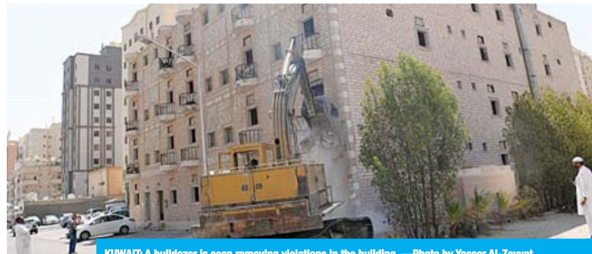
KUWAIT: A bulldozer is seen removing violations in the building. —Photo by Yasser Al-Zayyat
