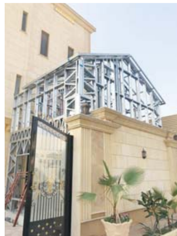
Galvanized steel is used to add a second floor at a house in Kuwait.
