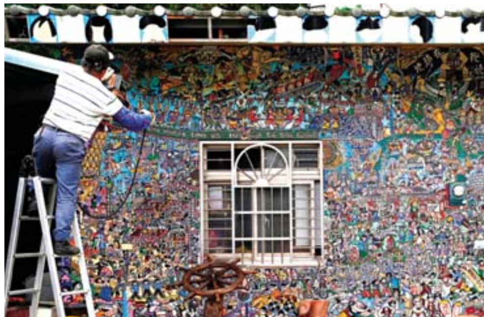
A man repairing a home which was painted by Hakka graffiti artist Wu Tsun-hsien in the Taiwanese village of Ruan Chiao.
