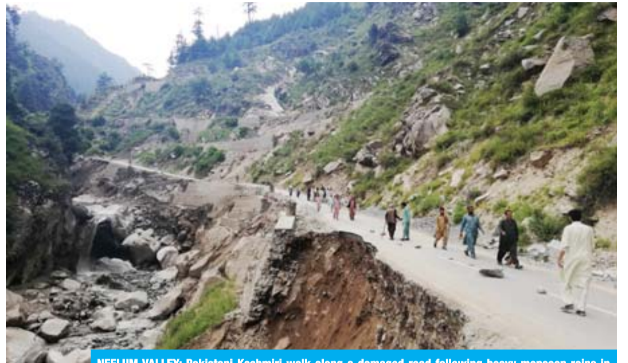
NEELUM VALLEY: Pakistani Kashmiri walk along a damaged road following heavy monsoon rains in Neelum valley near the Line of Control in Pakistan-controlled Kashmir yesterday. — AFP
