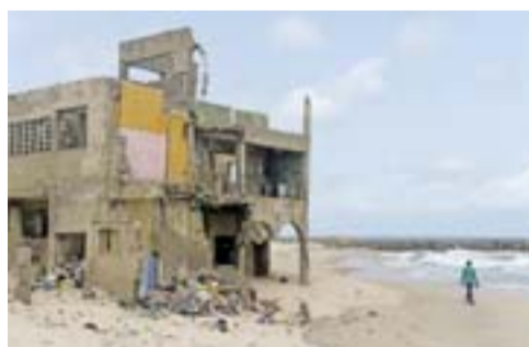
A man walks past an abandoned house destroyed by tidal erosion at Alpha Beach, a strip of the Lagos coastline, on April 29, 2019. — AFP
