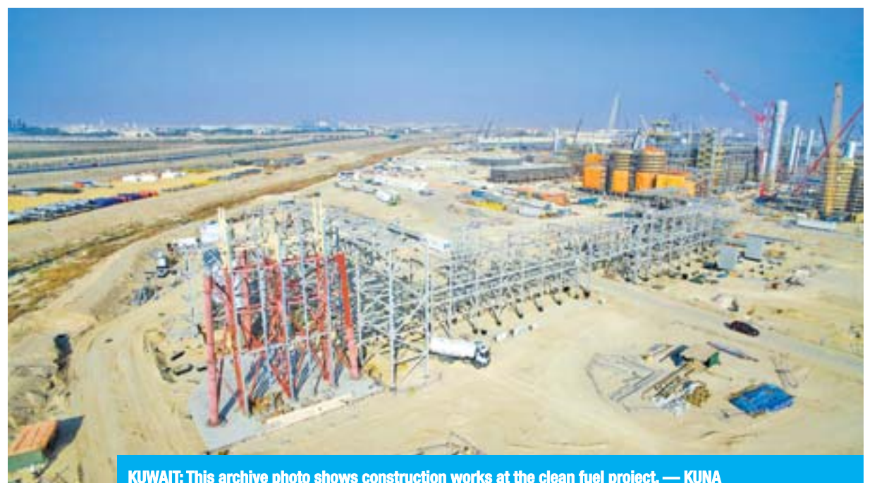
KUWAIT: This archive photo shows construction works at the clean fuel project. — KUNA
