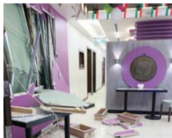
KUWAIT: Damage seen inside the Jahra restaurant following the explosion.
