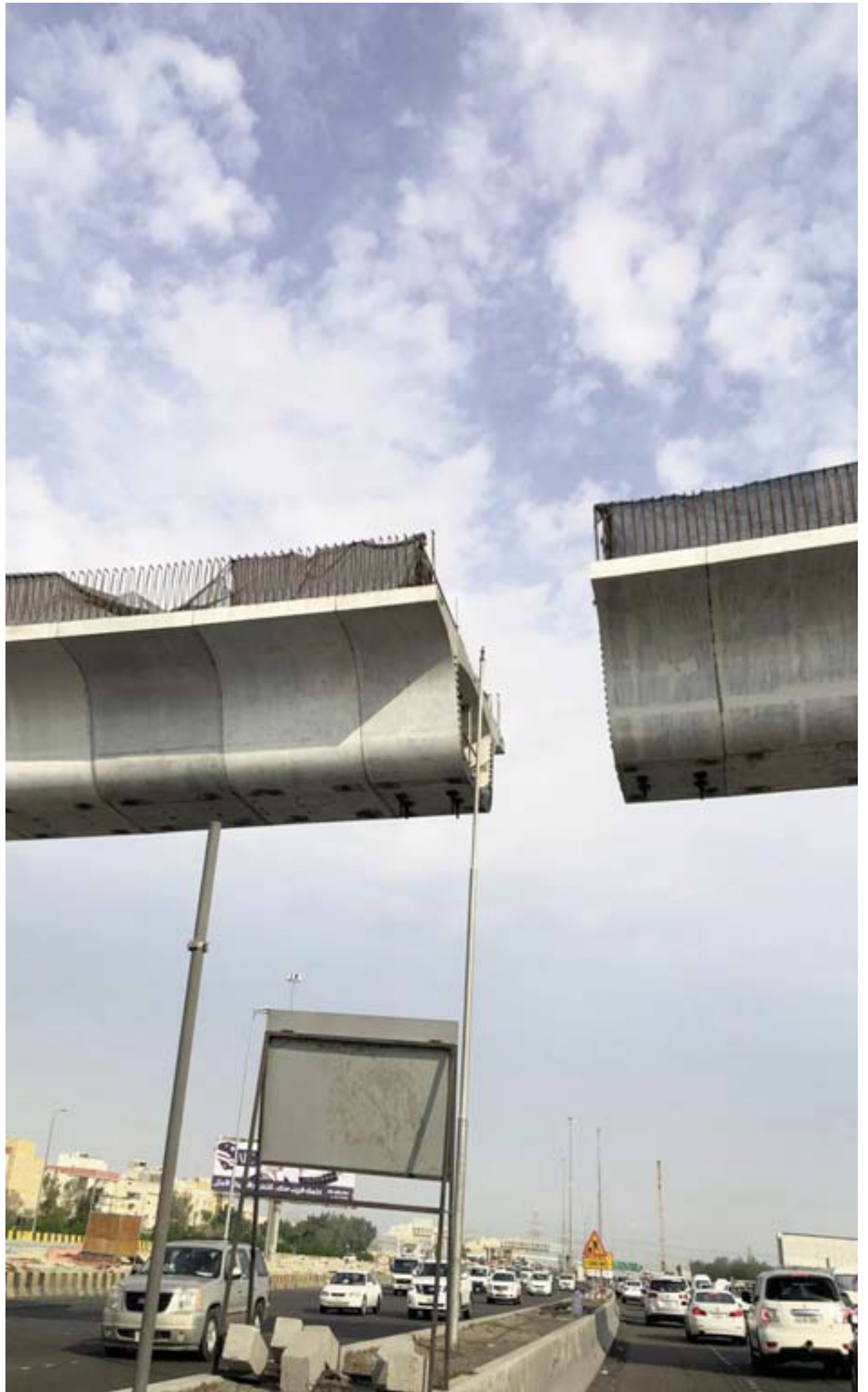
Almost there. A bridge over the 6th Ring Road reaches the final stage of construction. — Photo by Thomas Joseph
