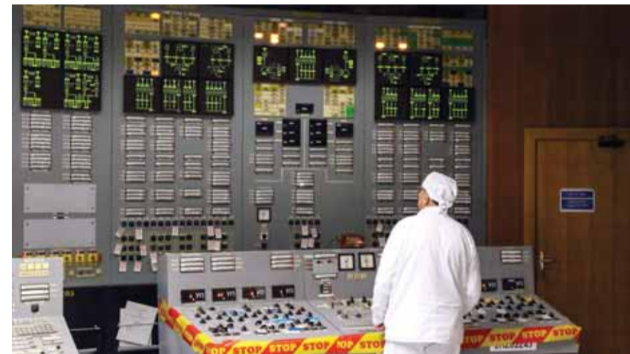
A man stands inside the monitoring room inside the inoperative Ignalina nuclear power plant in Visaginas, Lithuania.
