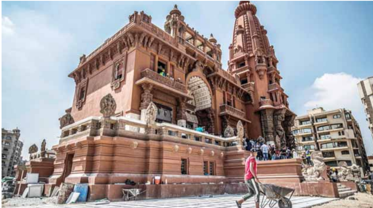
CAIRO: This picture taken on Sunday shows restoration works ongoing at the historic "Le Palais Hindou" (also known as the "Baron Empain Palace") in the Egyptian capital's Heliopolis district. — AFP
