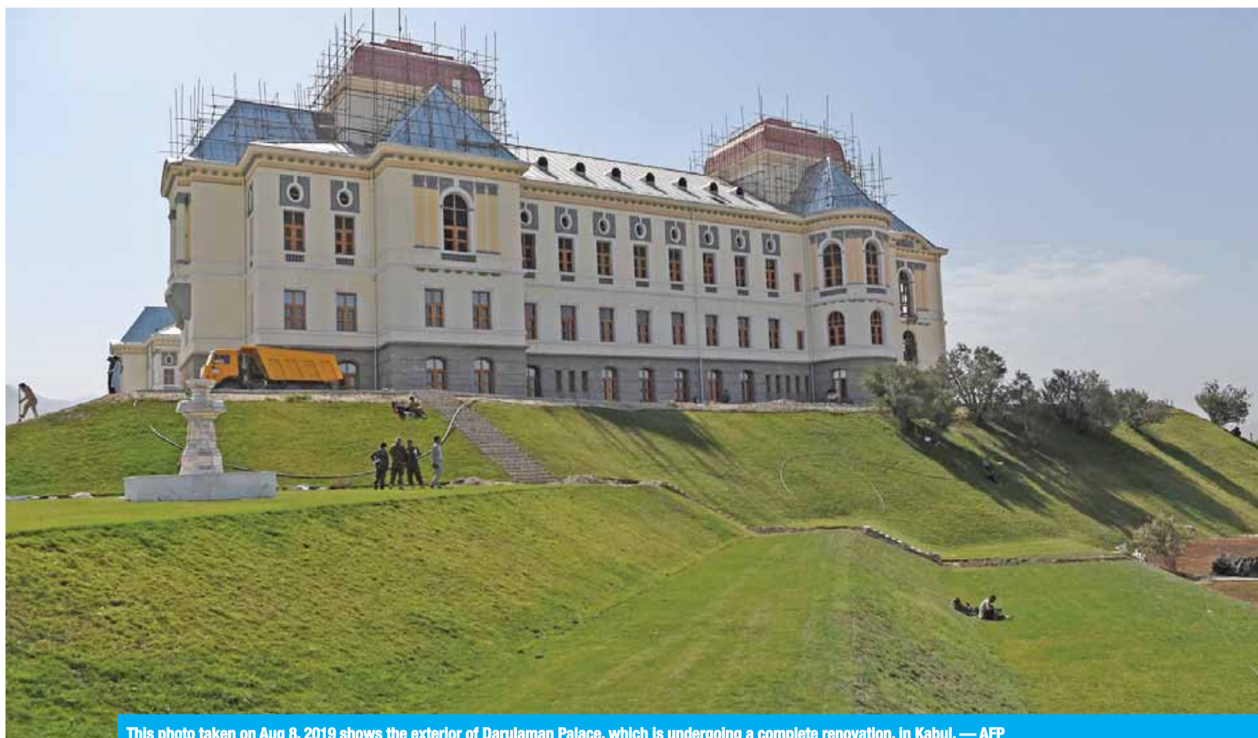
This photo taken on Aug 8, 2019 shows the exterior of Darulaman Palace, which is undergoing a complete renovation, in Kabul. — AFP
