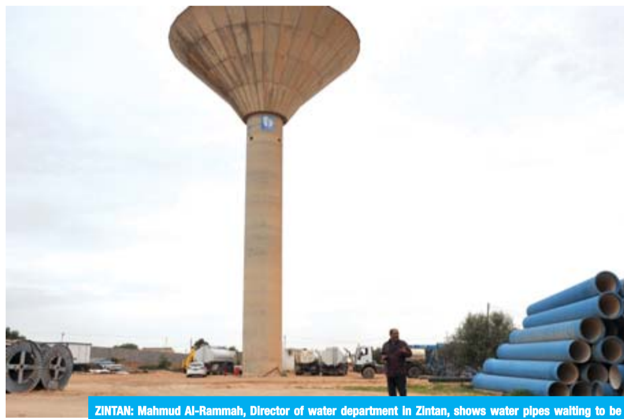
ZINTAN: Mahmud Al-Rammah, Director of water department in Zintan, shows water pipes waiting to be installed at the Zintan water pumping station in the city of Zintan. — AFP
