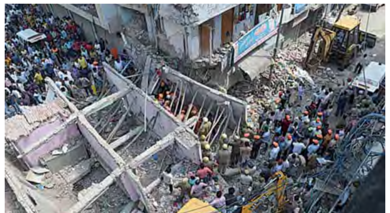
NEW DELHI: Members of the National Disaster Response Force (NDRF) search for victims after a building collapsed in New Delhi yesterday. —AFP
