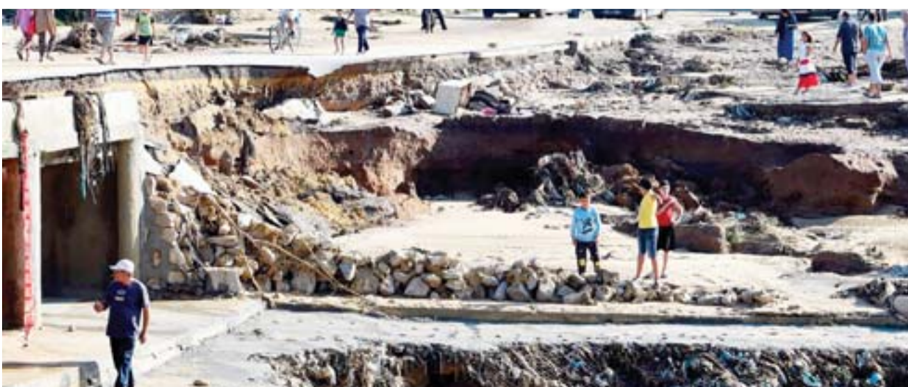
NABEUL, Tunisia: A picture taken yesterday in the Tunisian coastal governate of Nabeul shows people gathering at the site of collapsed bridge following deadly flash flooding in the town of Bir Challouf. — AFP
