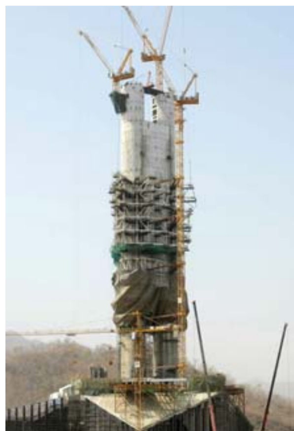
SARDAR SAROVAR DAM: Photo shows the under-construction 'Statue Of Unity' - a monument dedicated to Indian independence leader Sardar Vallabhbhai Patel, overlooking the Sardar Sarovar Dam near Vadodara in India's western Gujarat state. — AFP
