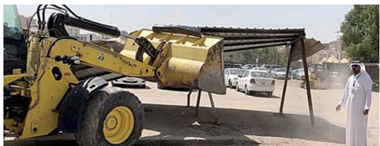
A municipality worker looks on as a bulldozer removes an unlicensed car parking shade during a recent campaign in Hawally.
