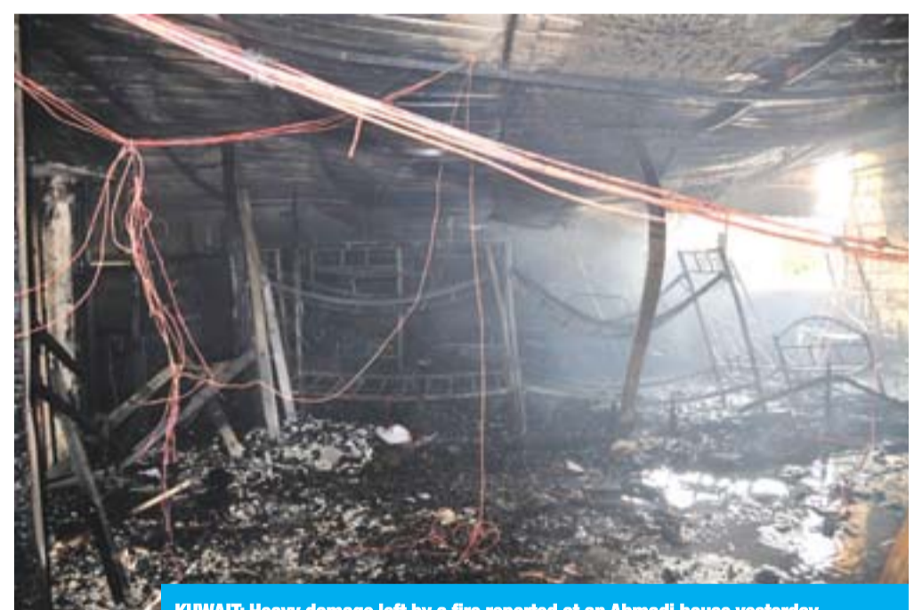
KUWAIT: Heavy damage left by a fire reported at an Ahmadi house yesterday.
