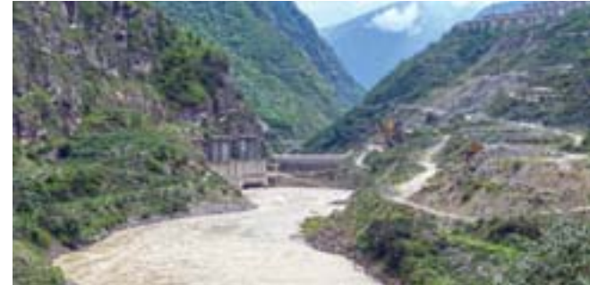
The Punatsangchu River flows into the first unit of the hydropower project, next to the under-construction site of the Punatsangchu hydropower project second unit, in Wangdue Phodrang.
