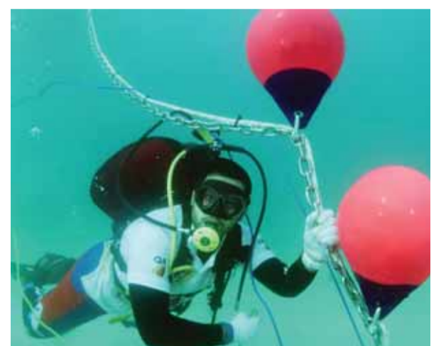
KUWAIT: Kuwait Dive Team affiliated with the Environmental Voluntary Foundation replaces and install cables on the island of Kubbar as part of a maintenance project. — KUNA photos
