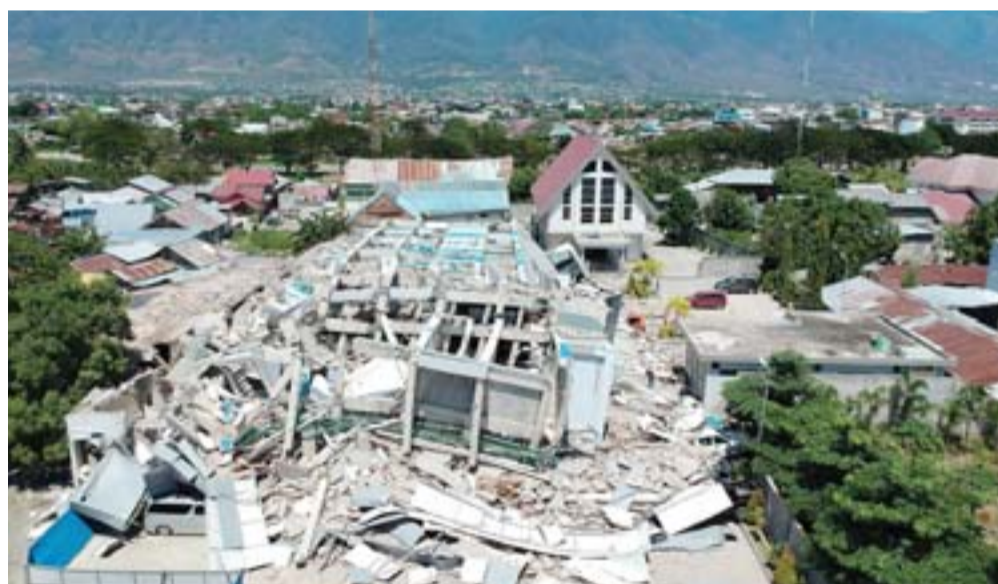
PALU, Indonesia: This aerial picture shows the remains of a ten-storey hotel in Palu in Indonesia's Central Sulawesi yesterday after it collapsed following a strong earthquake in the area. —AFP
