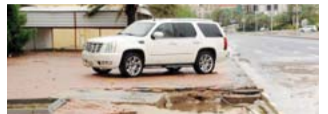
KUWAIT: This archive photo shows a damaged sidewalk pictured following the recent rainstorms. — KUNA
