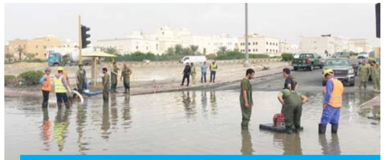
Ministry of Defense personnel help drain water from a submerged street.
