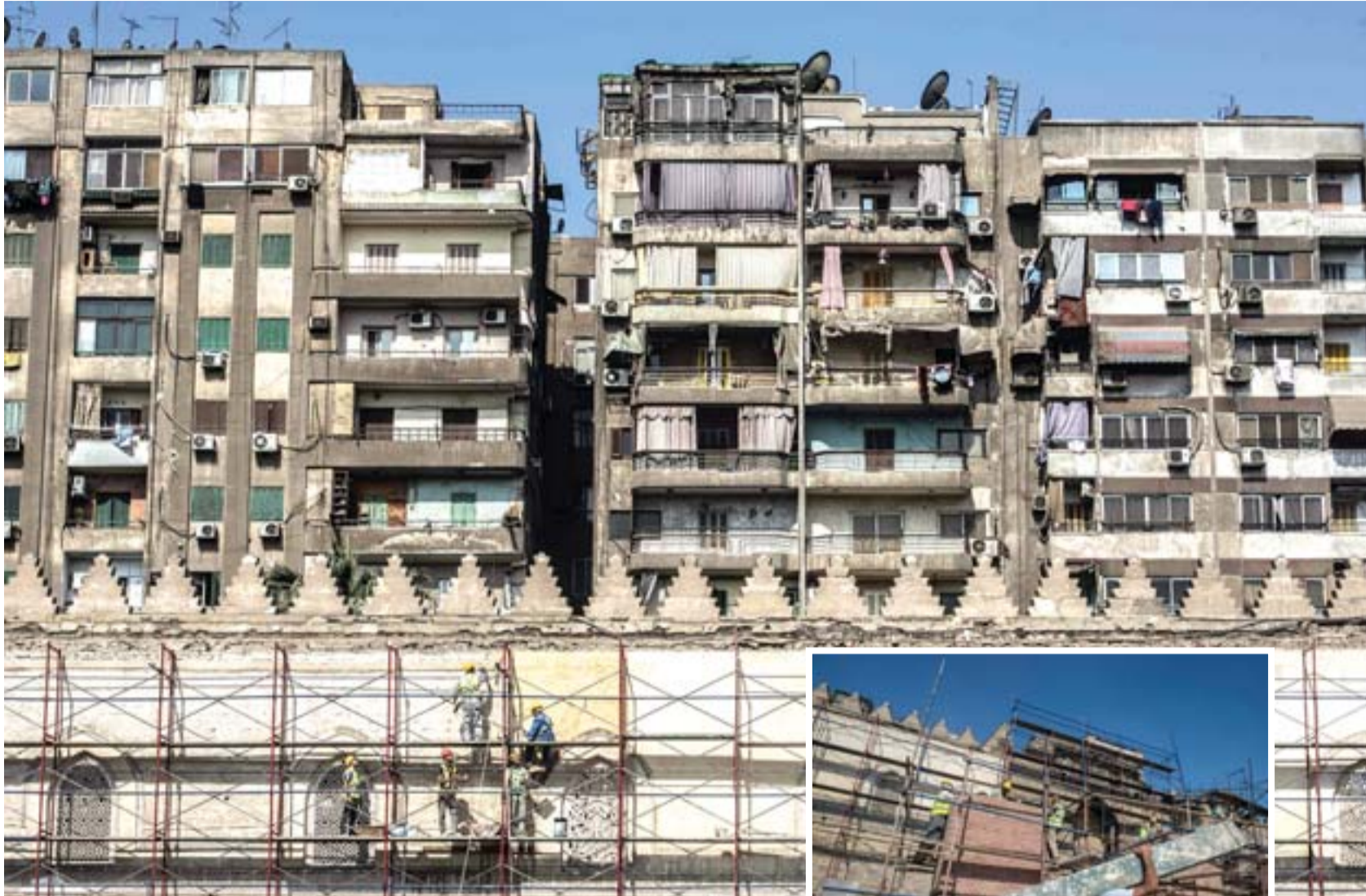
These pictures show workers standing on scaffolding during renovation work on the 13th century al-Zahir Baybars mosque in the capital Cairo. — AFP photos
