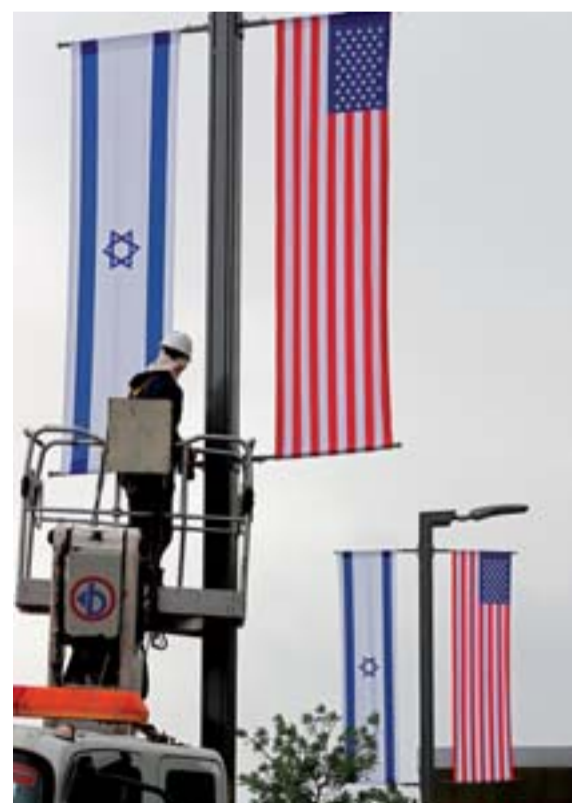
JERUSALEM: A worker installs decorations of Israeli and US flags in front of the US Consulate in Jerusalem where US officials will install the new US Embassy. The embassy move from Tel Aviv to Jerusalem is expected to occur on May 14. —AFP
