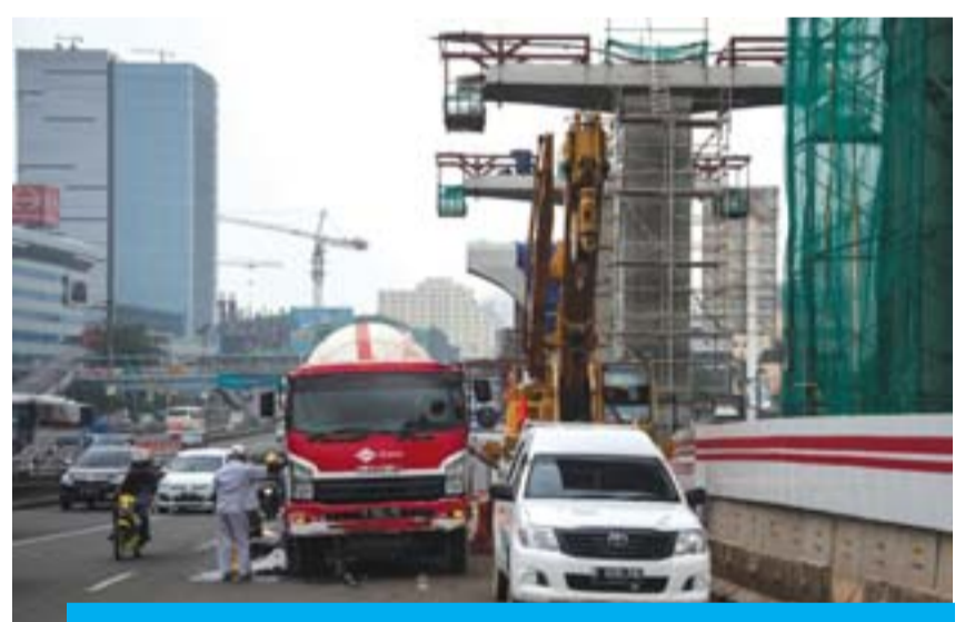
JAKARTA: This photograph shows a flyover for the light rapid transit (LRT) system under construction in Jakarta. —AFP
