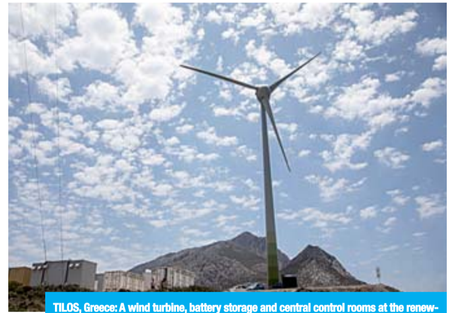
TILOS, Greece: A wind turbine, battery storage and central control rooms at the renewable energy "Tilos Project", are seen on the north coast of the Greek island of Tilos.
