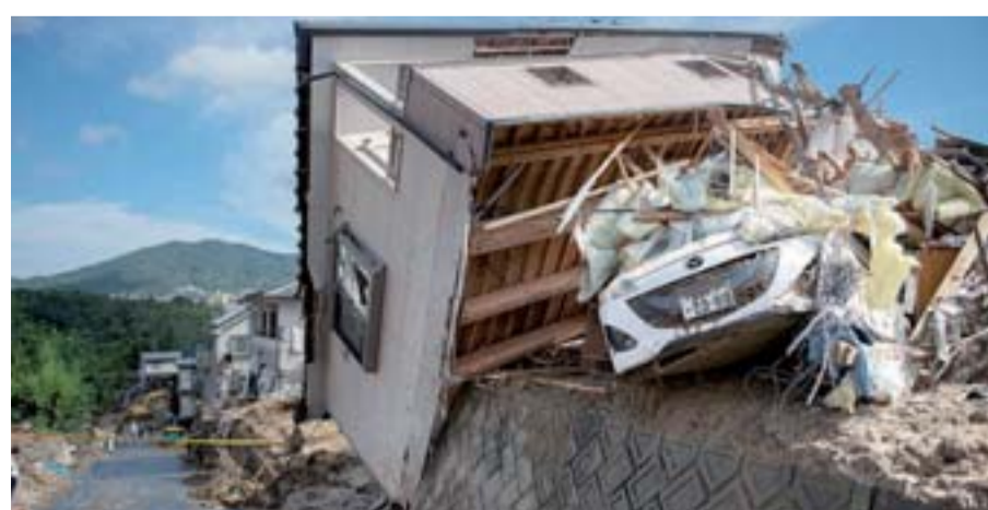
HIROSHIMA: This photo shows a damaged house in a flood hit area in Kumano, Hiroshima prefecture. —AFP
