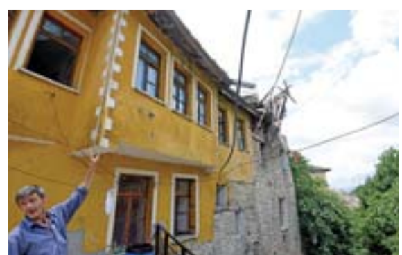
A man points to the damage to a house belonging to the Lolomani family in the UNESCO protected city of Gjirokastra.
