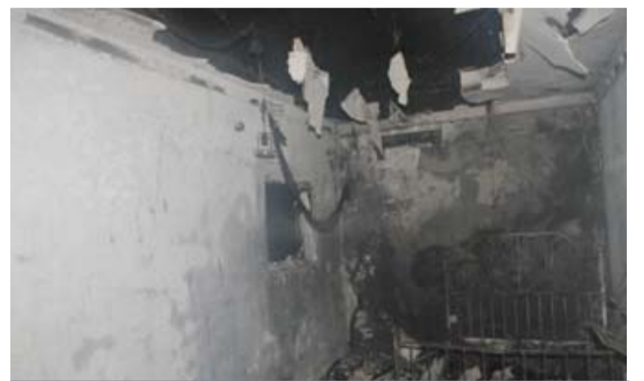
KUWAIT: Heavy damage caused by flames inside a Ferdous house where a fire was reported yesterday.
