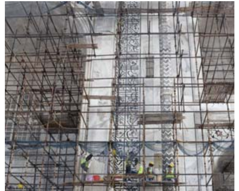
Indian laborers work amid scaffolding during conservation work at the Taj Mahal in Agra. — AFP photos
