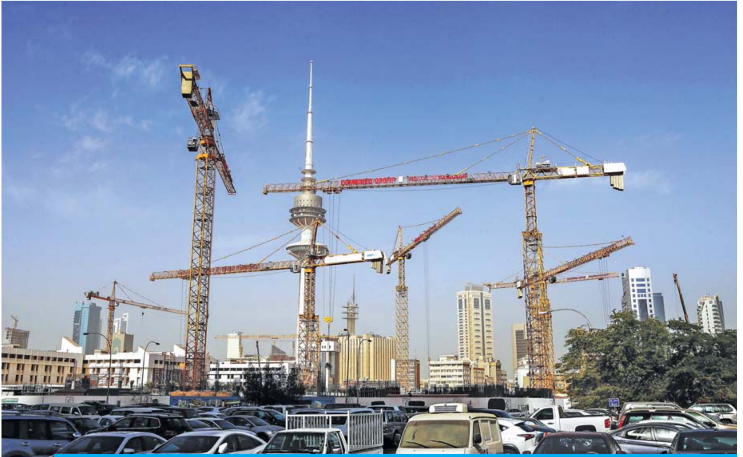
KUWAIT: A picture taken yesterday shows tower cranes operating at a construction site in Kuwait City with the 372-metre-high Liberation Tower seen in the background. — Photo by Yasser Al-Zayyat
