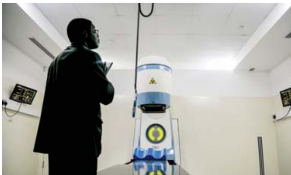
KAMPALA: A picture taken on January 19, 2018 shows a new Cobalt 60 Radiotherapy Machine being installed at Mulago hospital. — AFP
