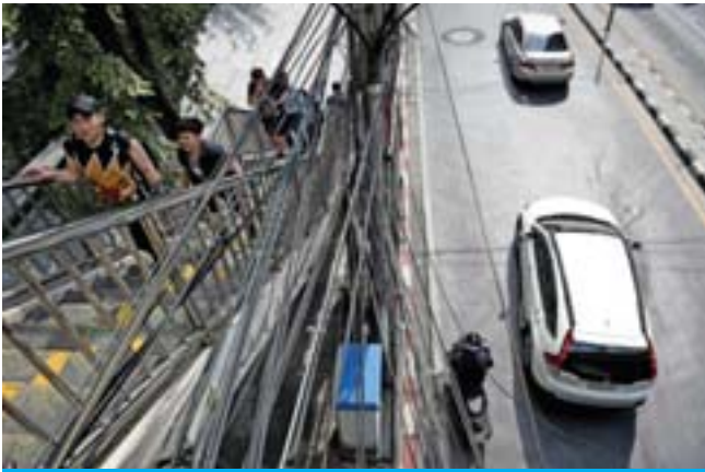
A network of cables strung along a crosswalk over Wireless Road in Bangkok.
