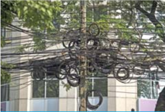
This photo shows a knot of cables hanging over Wireless Road in Bangkok. — AFP photos
