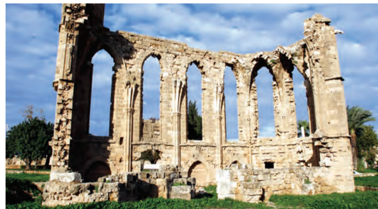
This picture shows the Saint George of The Latins Church, dating back to 14th century to be restored by the Technical Committee on cultural heritage in collaboration with UNDP and the European Union, in Famagusta, east of the self-proclaimed Turkish Republic of Northern Cyprus (TRNC). — AFP photos
