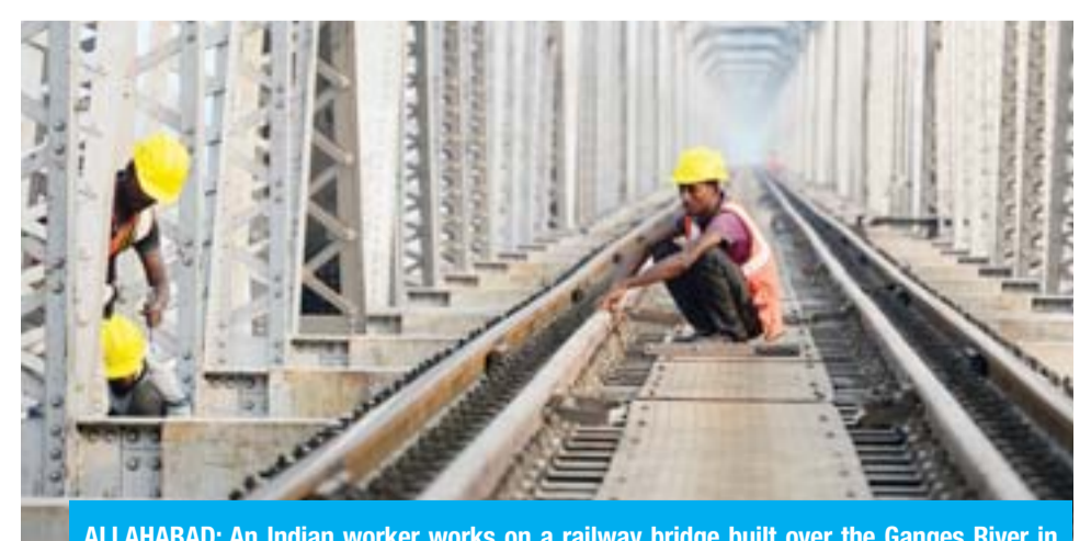
ALLAHABAD: An Indian worker works on a railway bridge built over the Ganges River in Allahabad yesterday. — AFP
