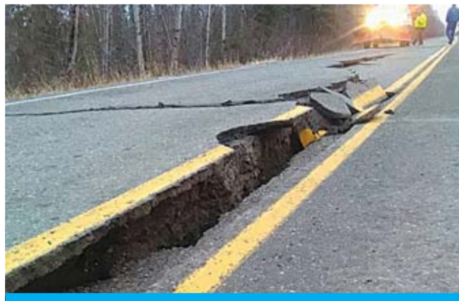
ALASKA: People walk past a crack in the road after an earthquake near Northwoods on the Kenai Spur Highway in Kenai, Alaska.—AFP
