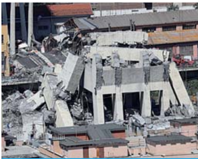
GENOA: This general view taken yesterday, shows the rubble of the collapsed section of the Morandi motorway bridge. —AFP
