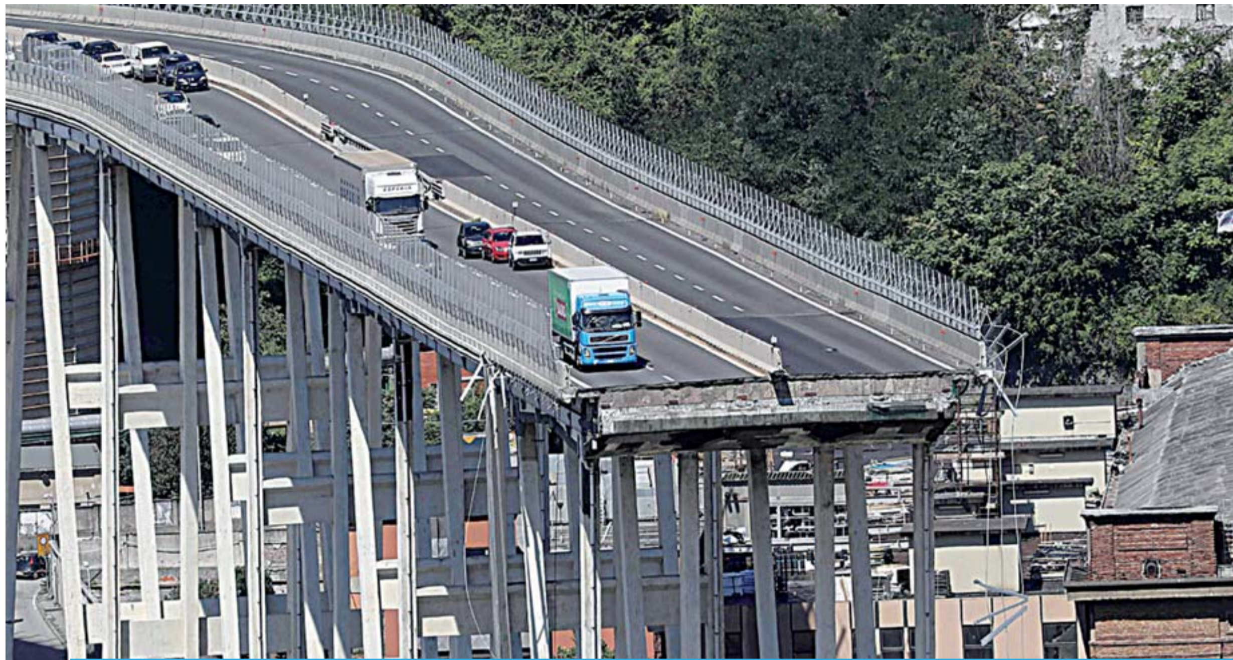
GENOA: This general view shows abandoned vehicles on the Morandi motorway bridge the day after a section collapsed in the north-western Italian city of Genoa. —AFP
