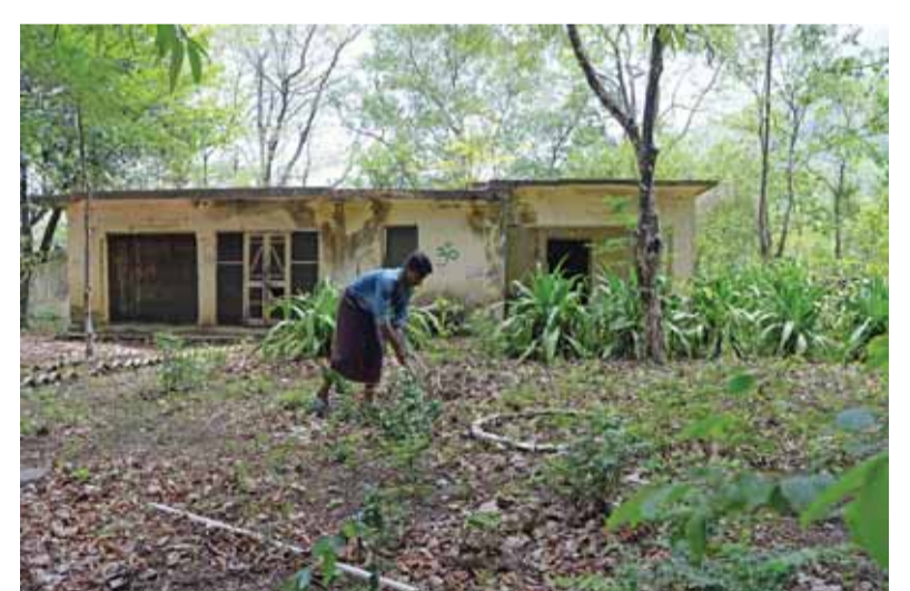
A worker clearing vegetation outside the former post office in the now-derelect ashram visited by the Beatles 50 years ago, in Rishikesh in northern India.
