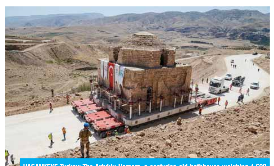
HASANKEYF, Turkey: The Artuklu Hamam, a centuries-old bathhouse weighing 1,600 tons, is loaded onto a wheeled platform and moved down a specially constructed road yesterday. — AFP
