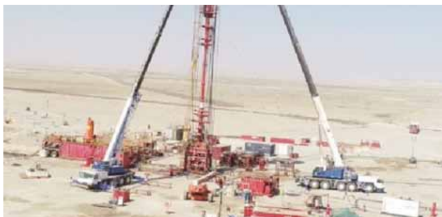
KUWAIT: This picture provided by Kuwait Oil Company shows works from the operation to contain oil leakage at Maqwa. — KUNA
