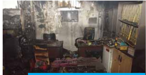
An office burned down by a fire reported at Shaab Cooperative Society yesterday.
